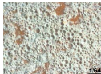
Excessive air voids are a common cause of low strength of concrete.
