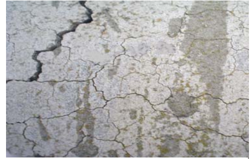
Fig: Map cracking of concrete can occur both by expansion and shrinkage mechanisms.
