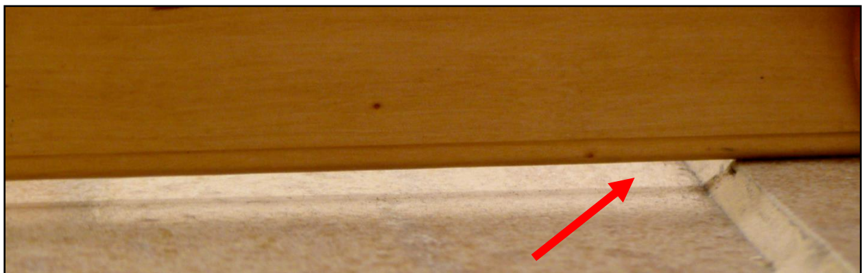
Example of extreme lippage on a tile floor installation
